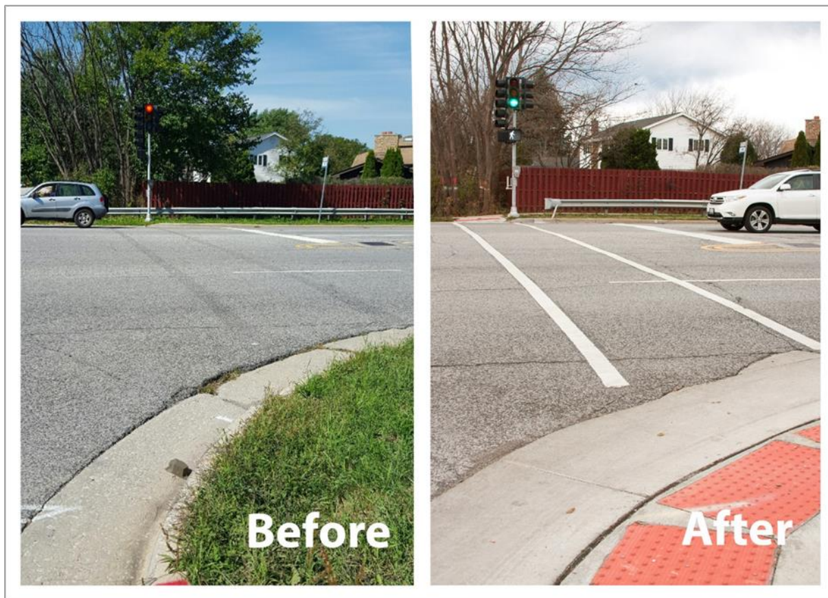
A new crosswalk at Harlem Avenue in Palos Heights provides better access to Pace's South Harlem route
